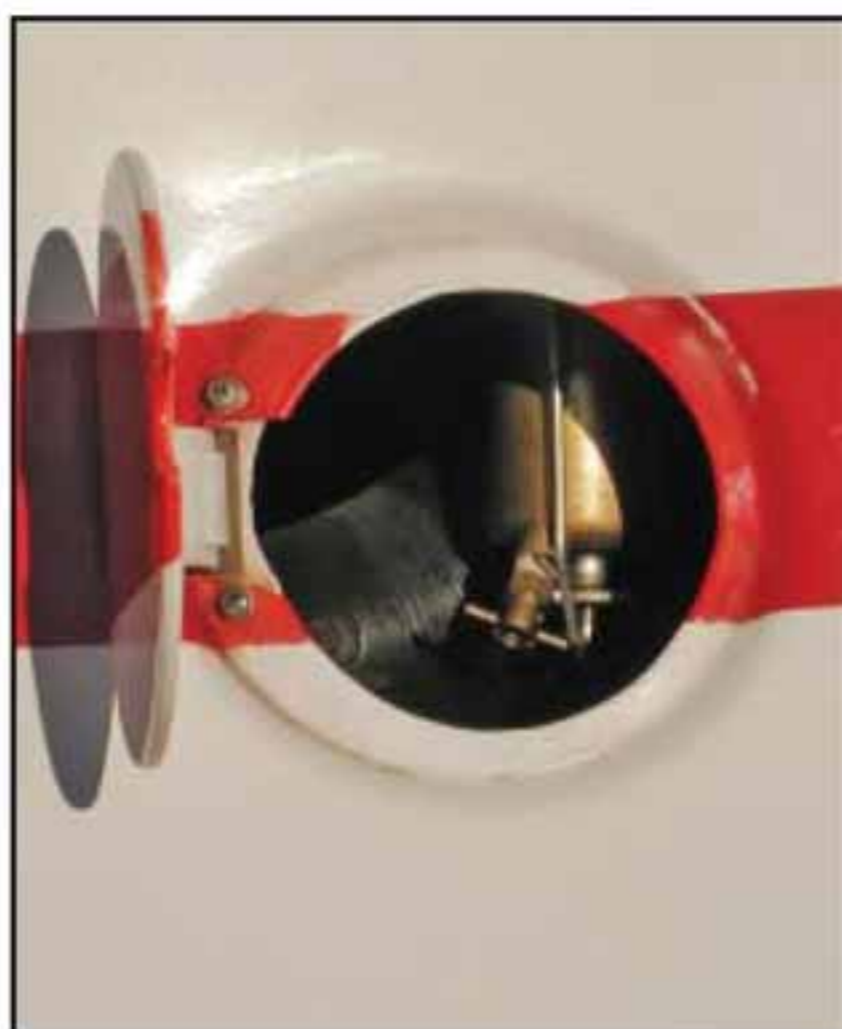
CLEAN DETAILS - Even the strainer drain is neatly tucked away behind a door similar to the fuel door on your car.
